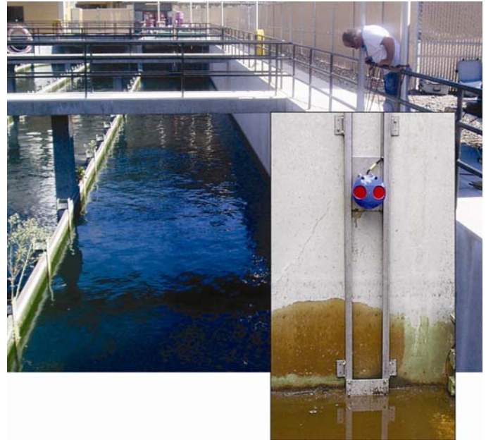
H-ADFM is well suited for monitoring flow in wide channels such as chlorine contact basins. Inset shows sensor mounting on vertical wall of basin.
