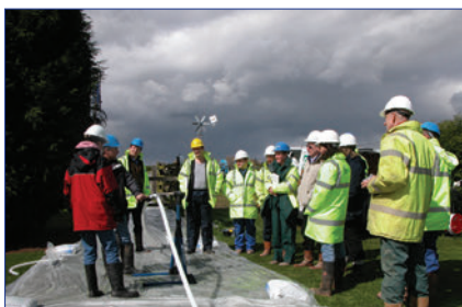
CMT Installation and training as part of a "Multilevel Course" given by the University of Cranfield at Silsoe, U.K., in conjunction with Waterra (UK), British Geological Survey & Norwest Holst.
