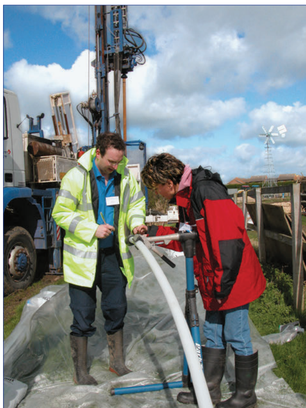
Construction of CMT ports in a 7-Channel system installed in Silsoe, England.
