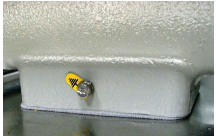
Figure 30: Earth ground connection
